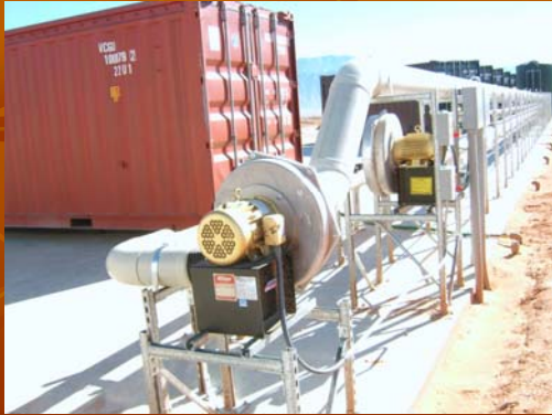
Positive and Negative Aeration System – Red Container is Biofilter
